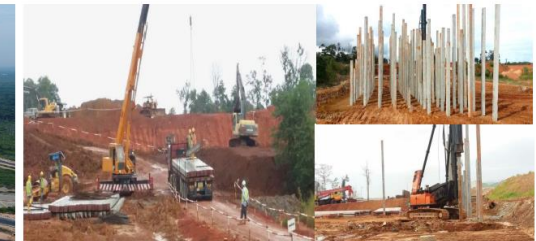
Extension of MCKIP Main Access Road to Northern Link Road 扩展北环路的主要通路
